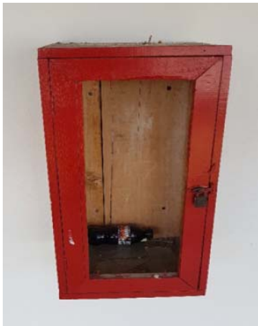
Empty Fire Extinguisher Holder
