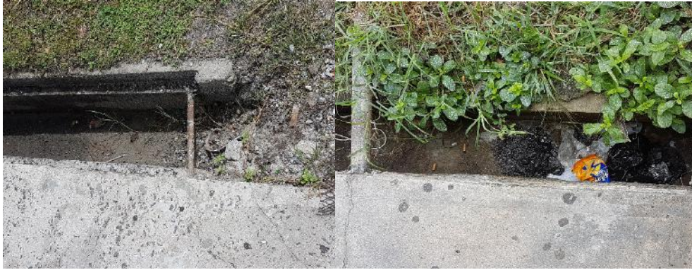
Garbage Filled and incomplete drains
