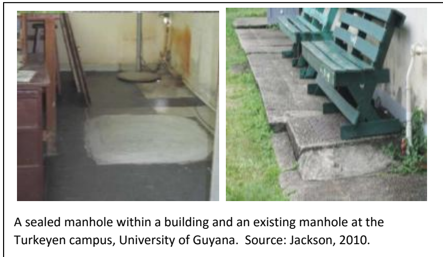
Figure 16 Manholes on Turkeyen Campus
