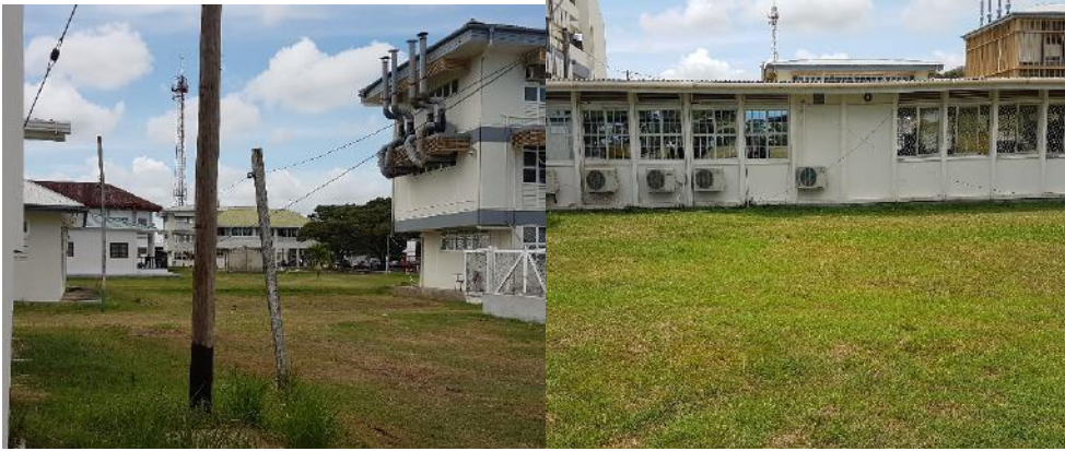
Low hanging wires close to the Faculty building and adjoining building
