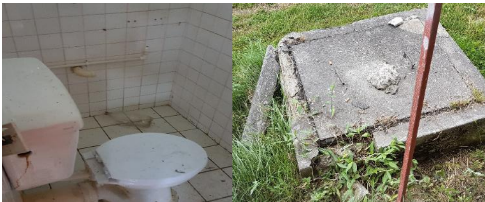
Unsanitary toilet and partially decaying septic system
